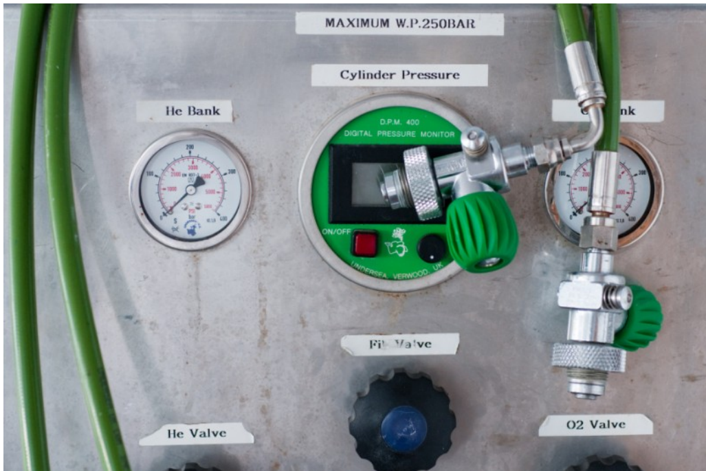
Compressors & Gauges on Whirlwind
